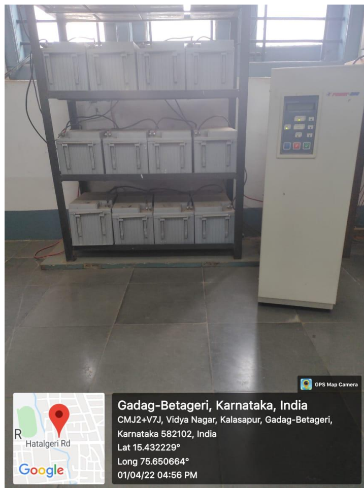
UPS of 6 kv
